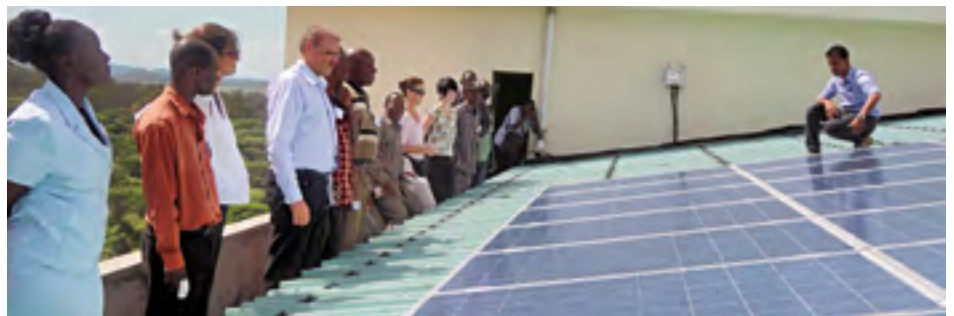
Lights back on for reading: solar panels installed on the roof at Saint Augustine University in Mwanza in 2010 generate enough electricity to illuminate the university library.
